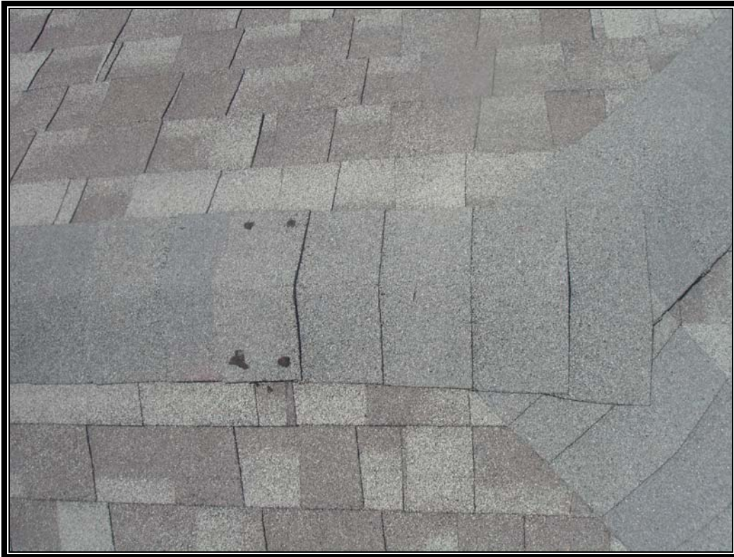
PHOTO #4: EXPOSED FASTENER - TYPICAL
