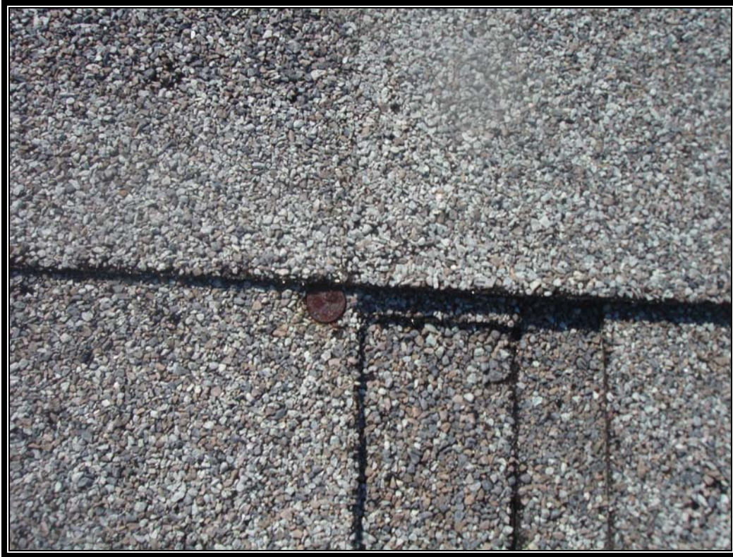
PHOTO #3: EXPOSED FASTENER – TYPICAL
